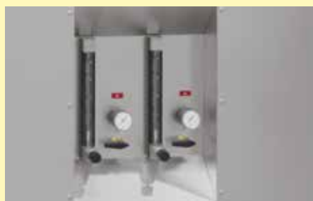
Automatic gas supply system
